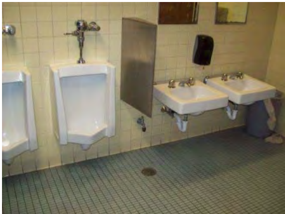
Photo #83: Typical restroom fixtures
