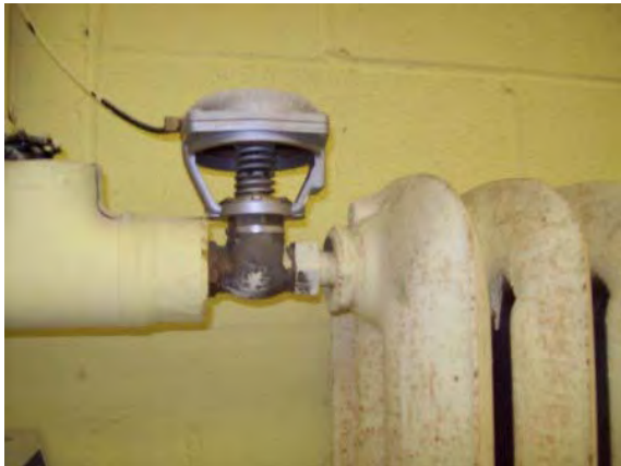
Photo #69: Steam radiator and pneumatic control valve
