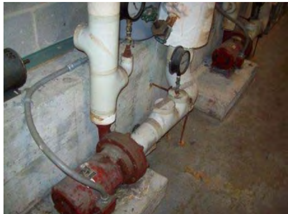
Photo #72: Chilled water circulating pumps
