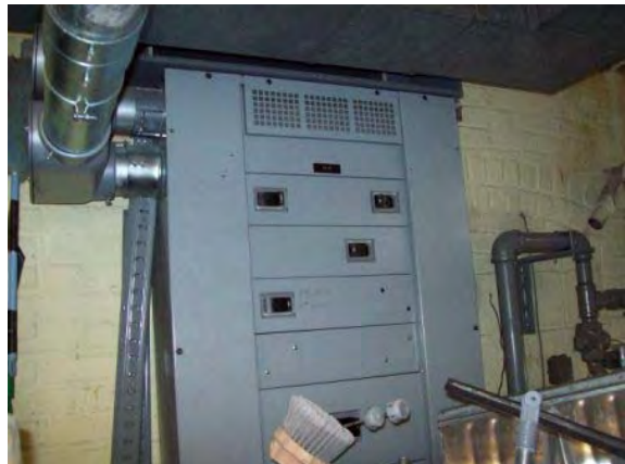
Photo #90: Main breaker panel
