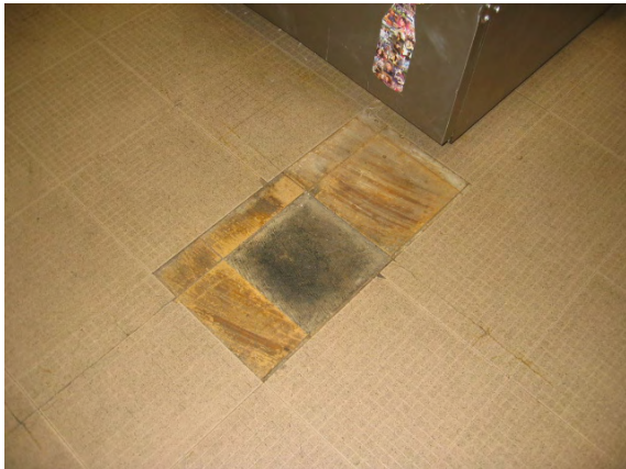
Photo #39: Poor conditions were observed at the kitchen VCT flooring
