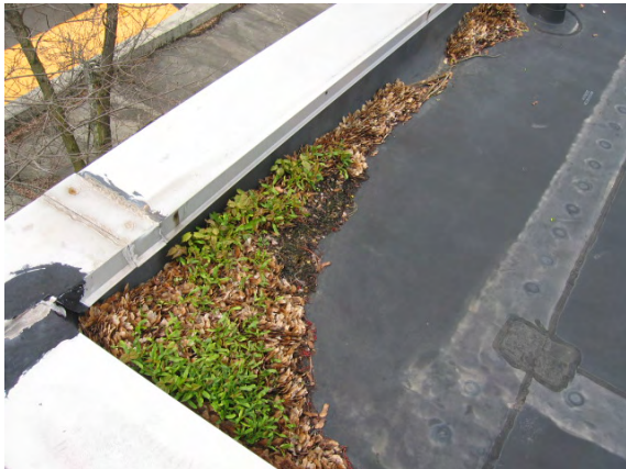
Photo #27: Several isolated sections of the roof debris and vegetation
