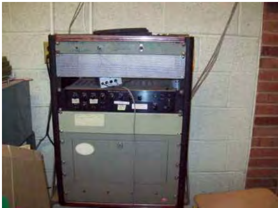
Photo #95: Auditorium sound system
