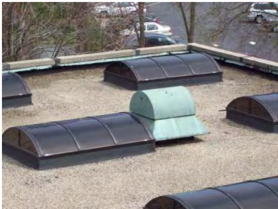
Photo #77: Gymnasium ventilation unit
