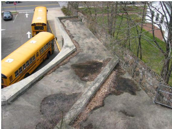
Photo #29: Carport canopy roof with fallen organic matter and ponding
