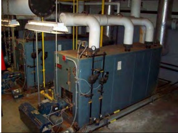
Photo #61: Steam boilers
