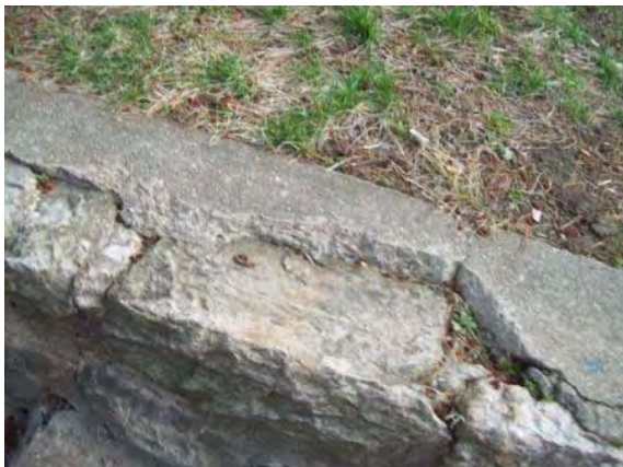
Photo #129: Damage at concrete steps
