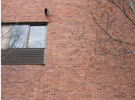
Photo #13: Portions of the brick facades have step cracking
