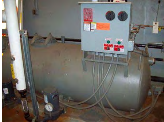
Photo #62: Condensate return system
