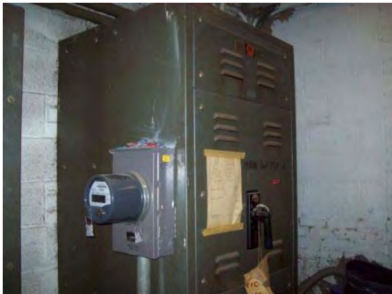
Photo #89: Electric meter and switchgear
