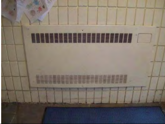
Photo #67: Recessed wall-mounted finned tube radiation heat unit
