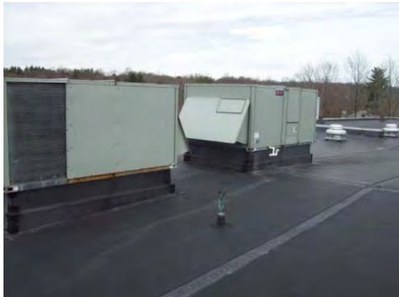
Photo #76: Rooftop package units
