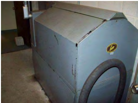
Photo #101: Hydraulic elevator equipment
