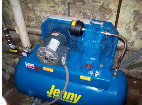
Photo #104: Compressor for dry sprinkler system
