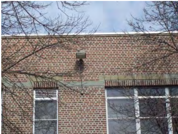
Photo #141: Building mounted site lighting
