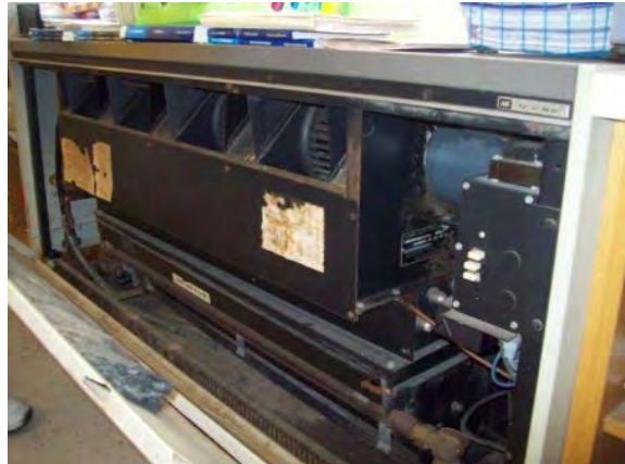
Photo #66: Unit ventilator with no cooling
