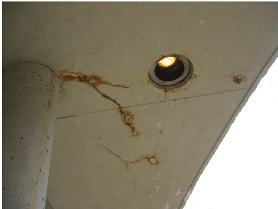
Photo #3: The carport canopy roof leaks frequently down through this light
