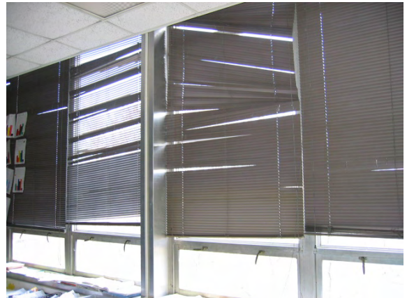
Photo #58: Many of the classroom window blinds are damaged and inoperable
