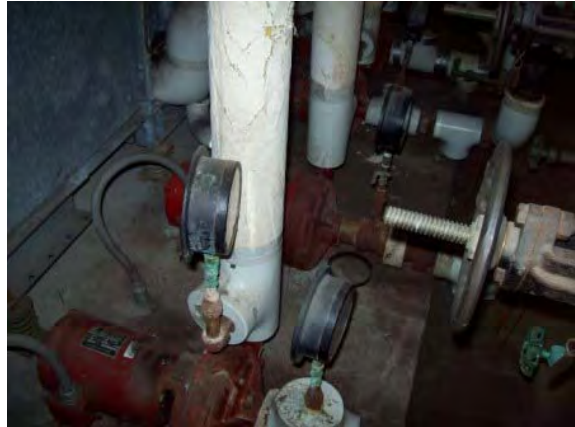
Photo #64: Hot water circulating pumps
