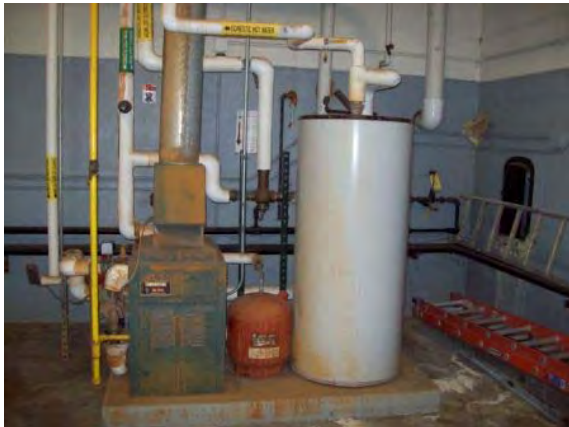
Photo #81: Domestic water boiler and storage tank
