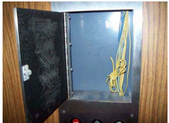
Photo #100: Missing emergency communication equipment
