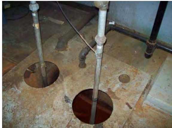
Photo #82: Sump pump
