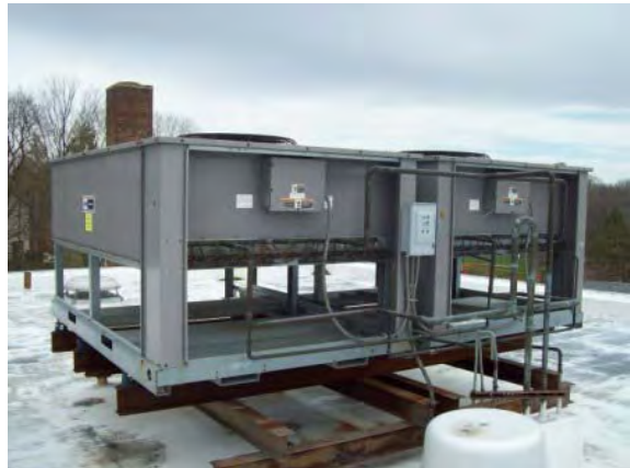
Photo #70: Air cooled condensing unit
