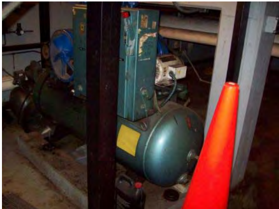
Photo #75: Compressor for pneumatic controls
