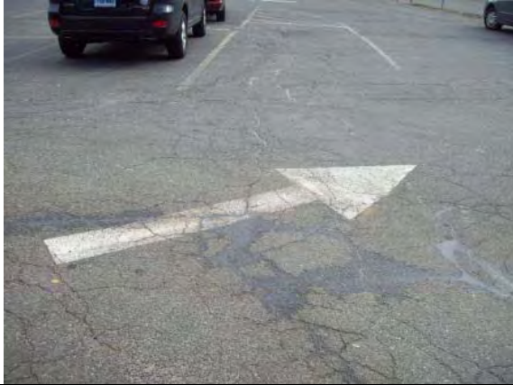
Photo #121: Asphalt damage in rear parking lot
