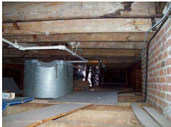
Photo #106: Sprinkler piping in attic
