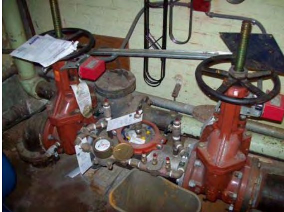
Photo #103: Fire sprinkler line and backflow preventer
