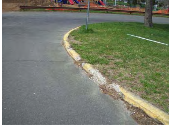
Photo #122: Curb damage in rear parking lot
