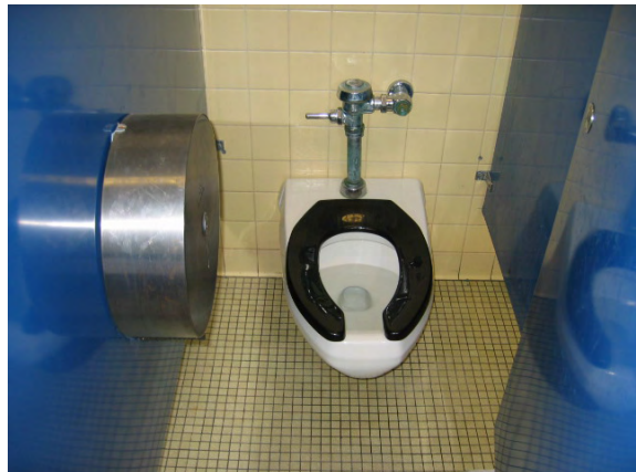
Photo #48: No grab bars are provided within the toilet stalls
