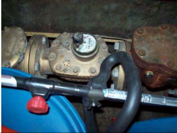
Photo #79: Domestic water meter
