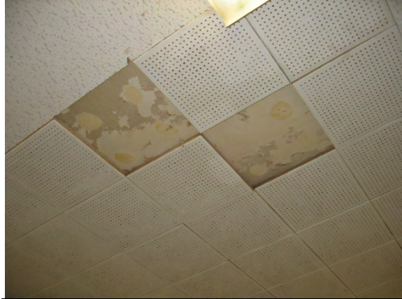
Photo #38: Poor conditions were observed at the adhered kitchen ceiling
