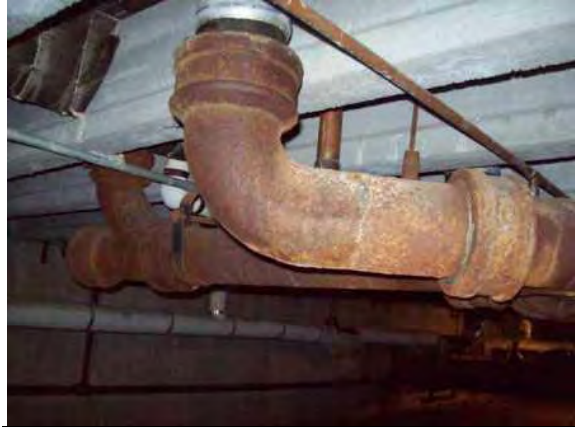
Photo #80: Typical sanitary waste lines
