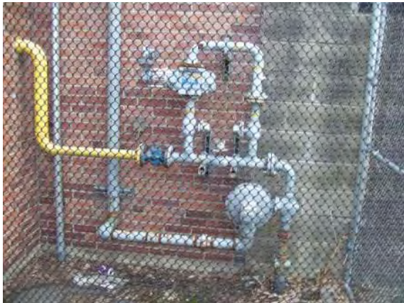
Photo #87: Gas meter and regulator
