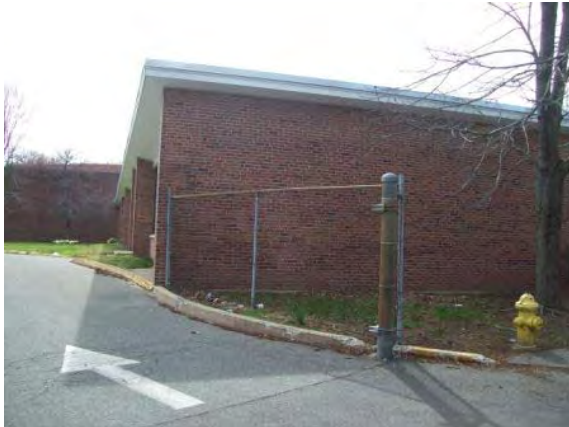
Photo #137: Corrosion at fencing near southeast corner of building
