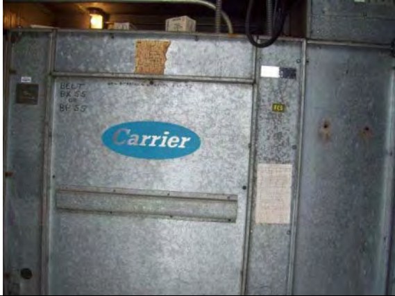
Photo #73: Air handling unit for office area (AC-1)
