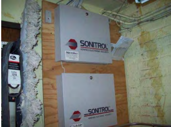
Photo #109: Security panels
