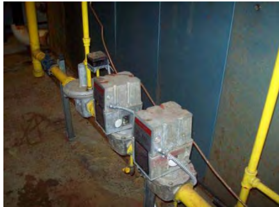
Photo #88: Gas feed for boiler
