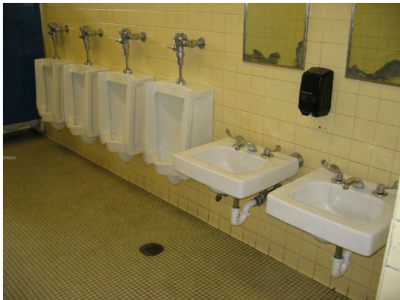
Photo #47: Typical multi-user common toilet room. Note the lack of ADA access
