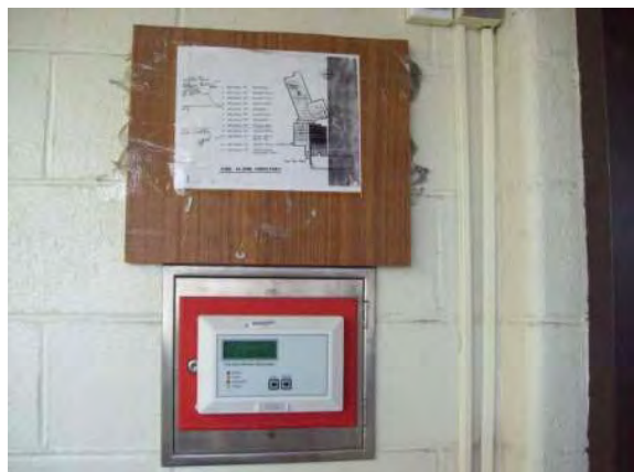
Photo #108: Fire alarm annunciator panel
