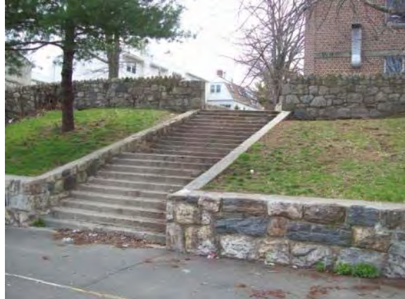
Photo #128: Concrete steps near play area without handrails
