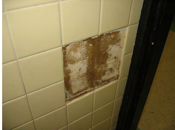
Photo #50: Several sections of the toilet room wall tiles in the primary section are damaged
