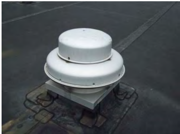
Photo #78: Typical exhaust fan
