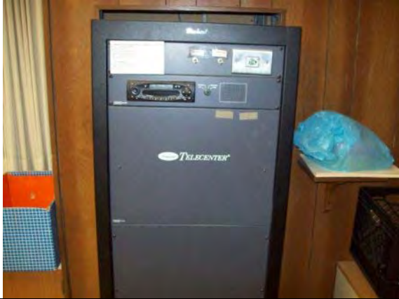
Photo #91: PA system control unit
