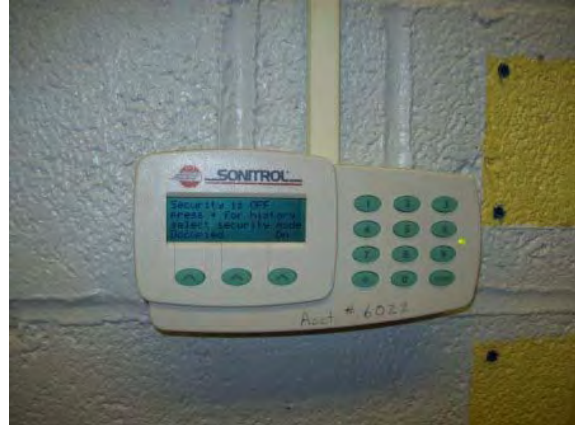
Photo #110: Security interface panel
