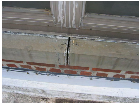
Photo #12: Portions of the window frames have open caulk joints
