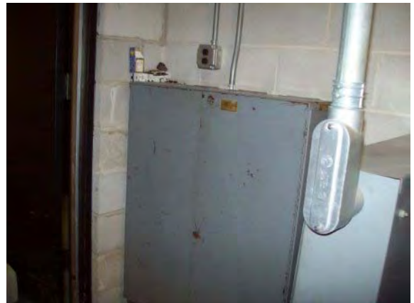
Photo #102: Elevator controller
