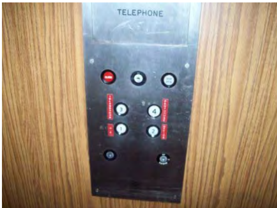
Photo #99: Elevator control panel
