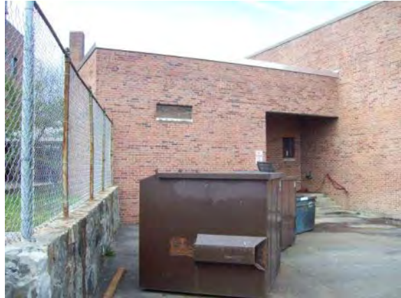
Photo #136: Corrosion at fencing near loading dock
