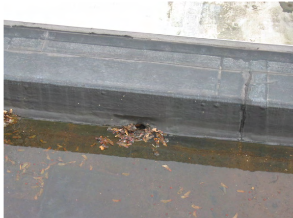
Photo #28: Several of the roof drain strainers are missing or clogged
