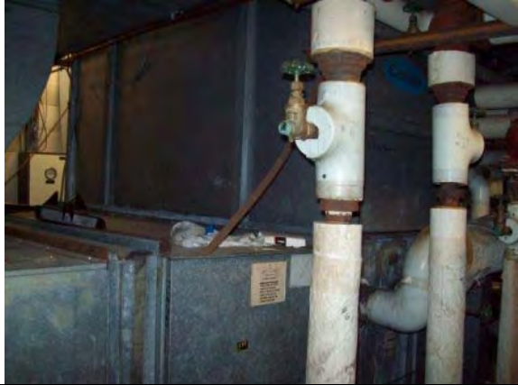
Photo #74: Air handling unit for media center (AC-2)
