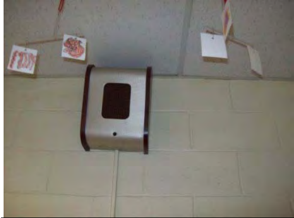
Photo #92: Typical PA speaker in classroom
