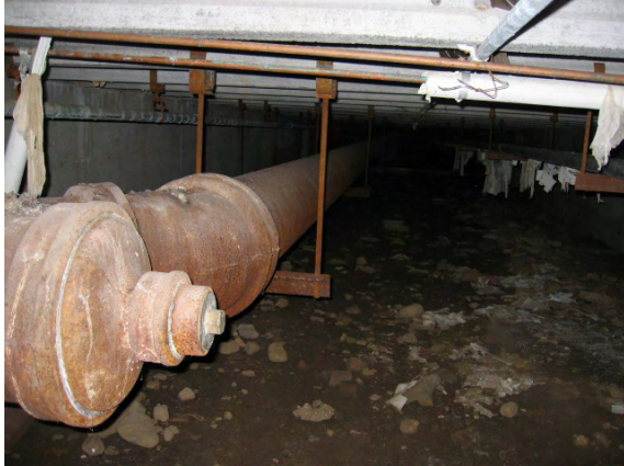
Photo #31: Chronic leaks were reported at the main roof drain main located in the crawl space
