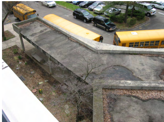
Photo #30: Carport repairs are required due to leaks
