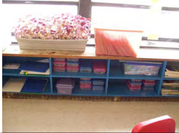
Photo #68: Cabinet mounted finned tube radiation unit
