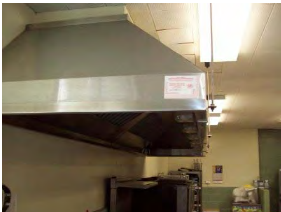
Photo #113: Exhaust hood with no Ansul system
