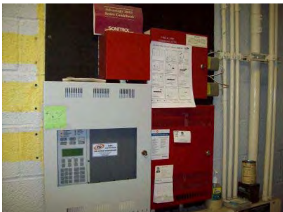
Photo #107: Fire alarm control panel
