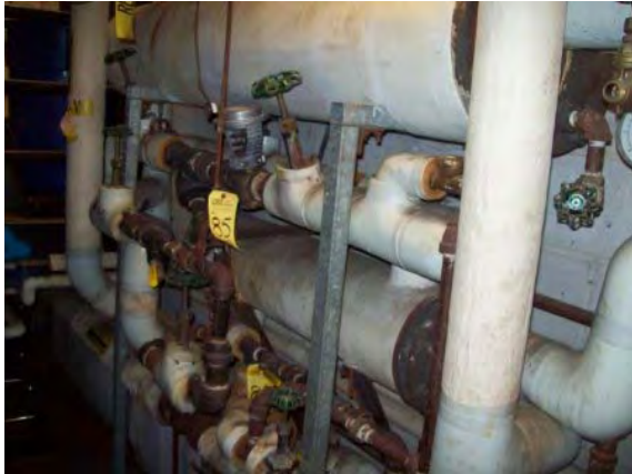
Photo #63: Heat exchangers
