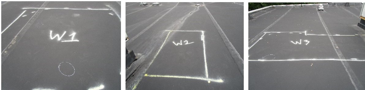
Wet areas in Roof A with holes marked
