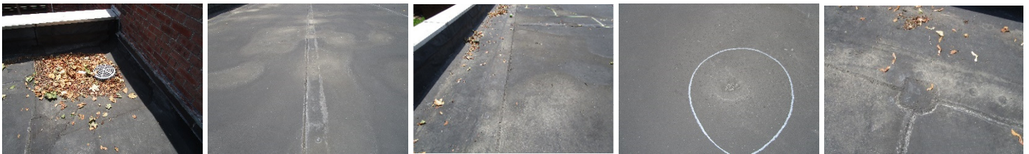
Debris clogging drains Worn and cracking lap Cracking lap Scrim visible thru membrane Cracking laps
