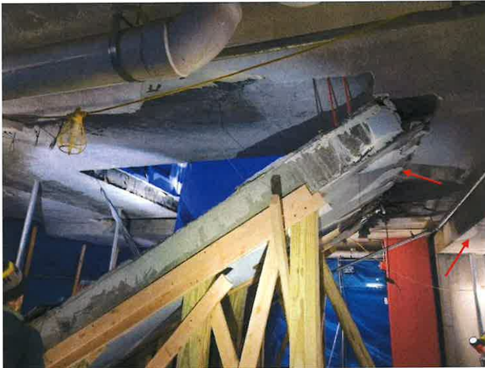
Figure 5- Shear Failure at West End. Note B21 Beam. Collapsed Area looking South
