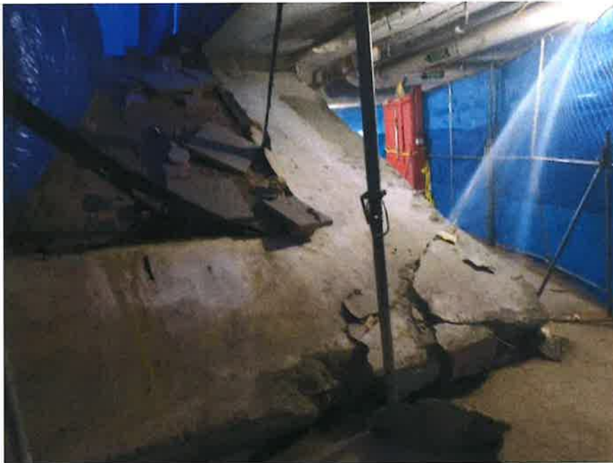
Figure 1- Partially Collapsed 5 th Level Slab. Looking East to West
