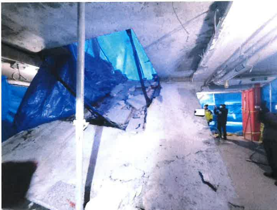
Figure 4- Partially Collapsed Slab looking West
