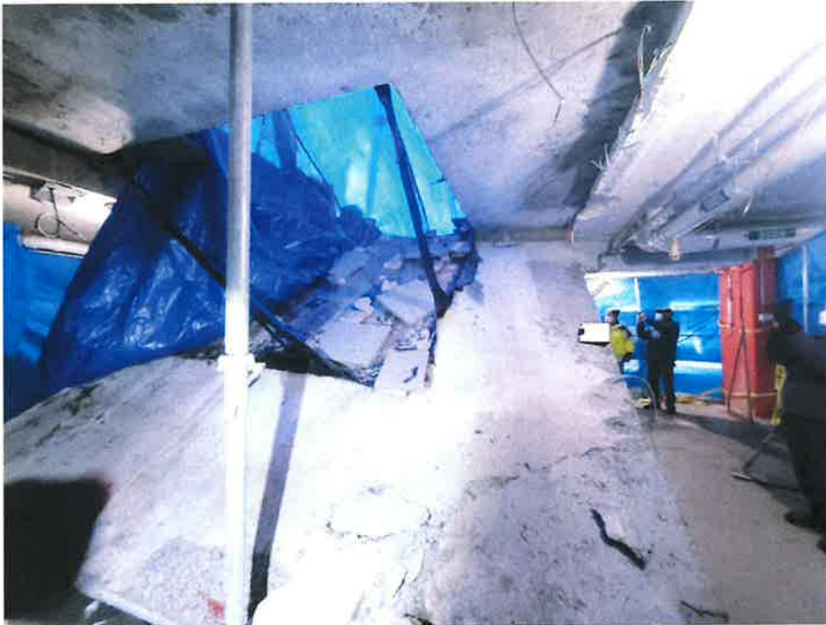
Figure 7- Partially Collapsed Slab looking West
