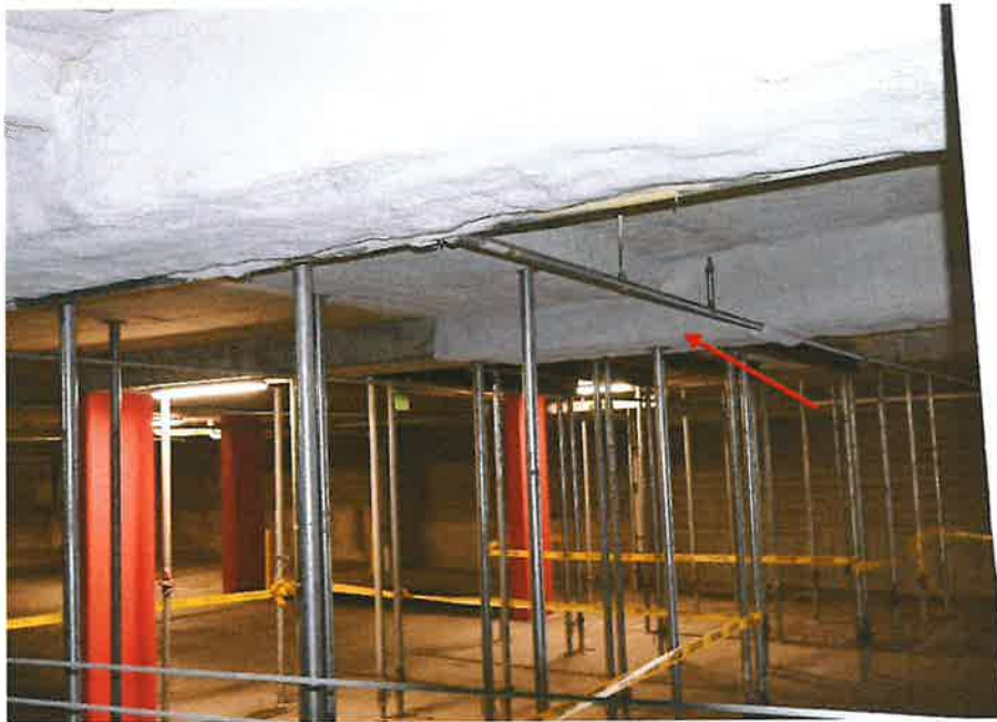
Figure 16- Added Beam Not Shown in any Drawings at Line GD (arrow)
