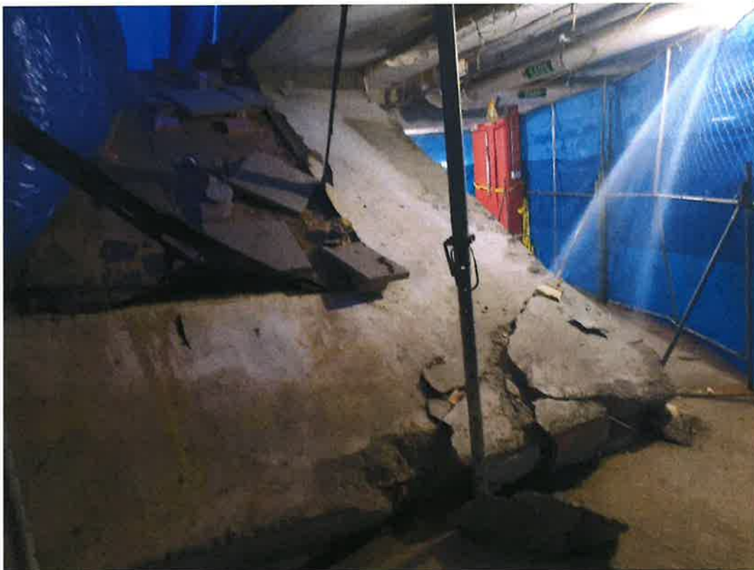
Figure 4- Partially Collapsed 5 th Level Slab. Looking East to West
