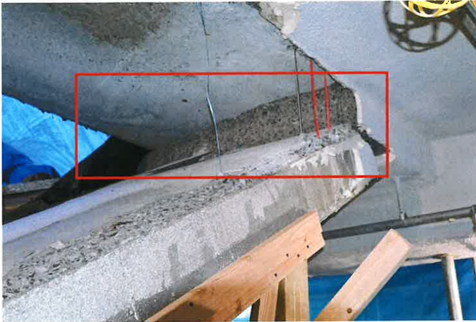
Figure 11- No top reinforcement at failure plane Northwest Portion of Collapsed Slab. Note smooth formed surface at underside of upper slab at transition.
