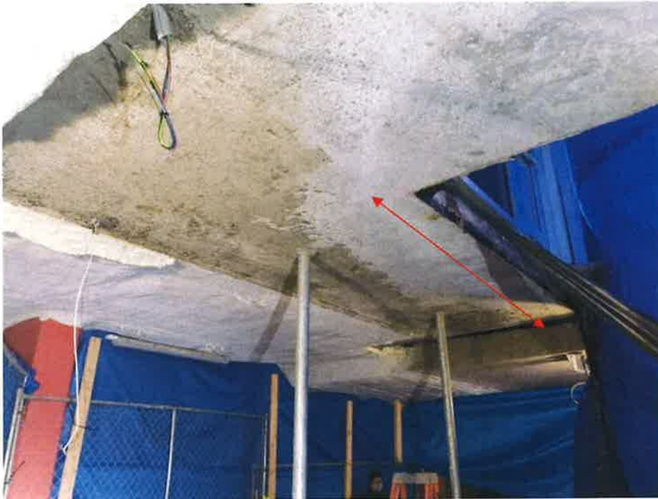
Figure 13- Upper Slab Reinforcement in the Area of the Collapsed Slab is Unknown.
