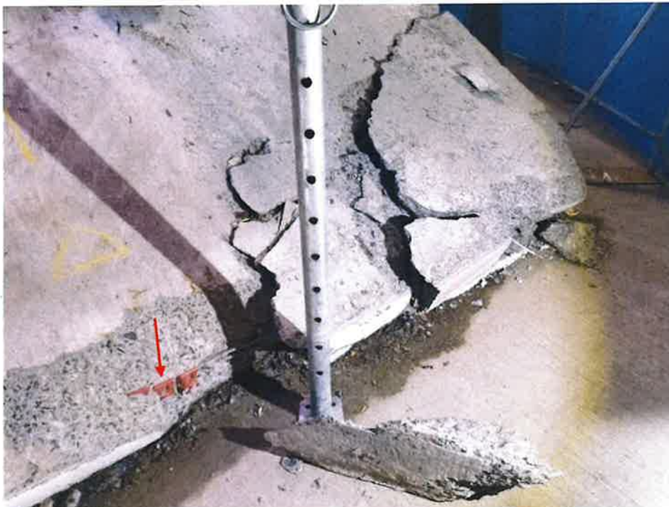
Figure 6- Live End Anchorages at East End of Lower Collapsed Slab
