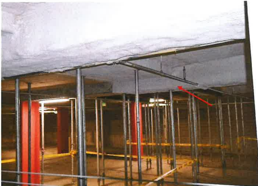
Figure 12- Added Beam Not Shown in Drawings at Line GD
