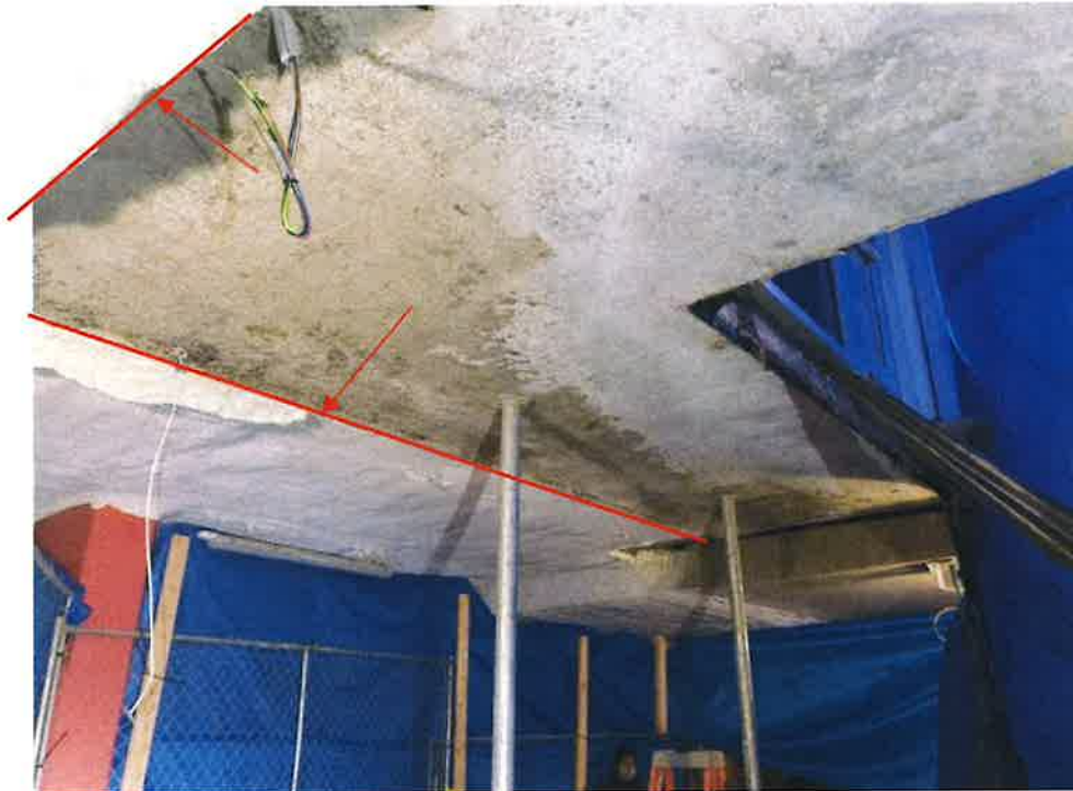
Figure 7- Construction Joint Between Upper and Lower Slab. East End of Collapsed Slab
