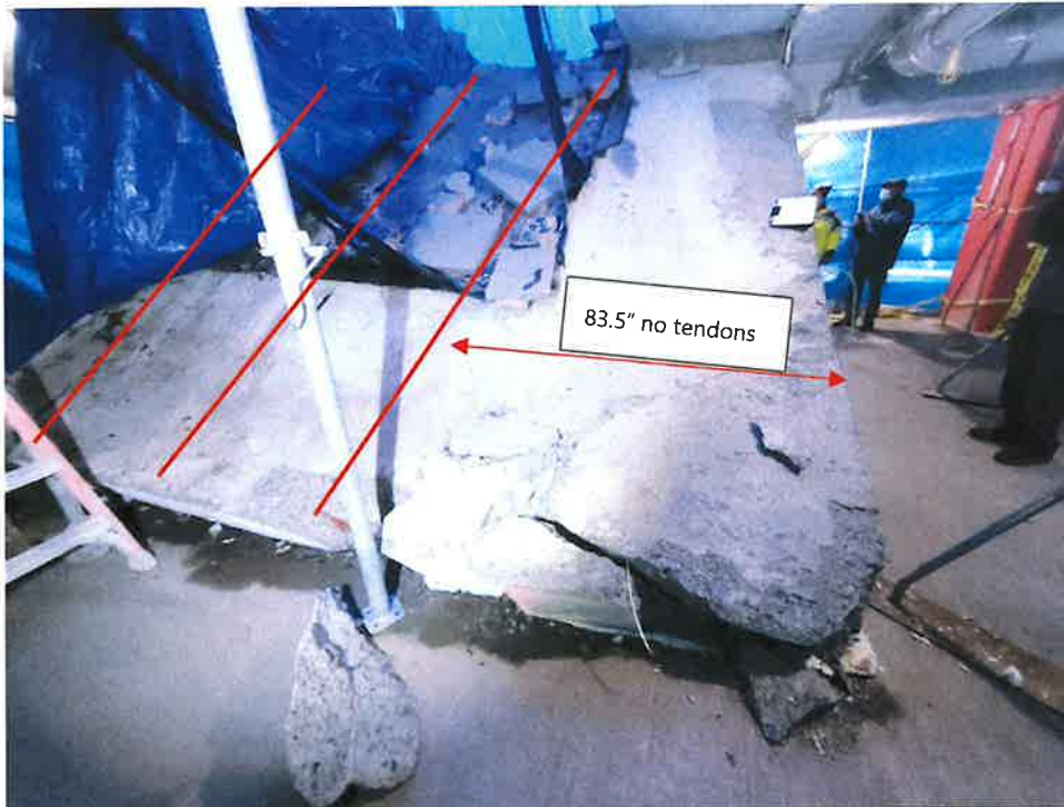
Figure 13- PT Layout at Slab Looking East to West. Red lines indicate positions of PT strands
