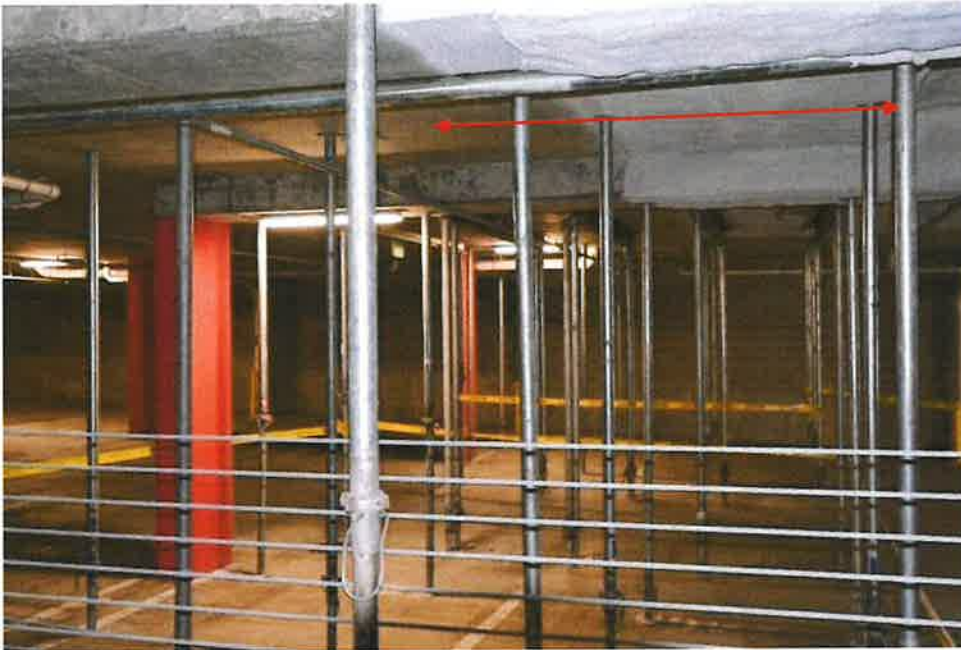
Figure 11- Lower Slab to West of Collapsed Portion. 83.5 in. area with No Tendons in Collapsed Area. Cannot Scan Cause of Insulation.
