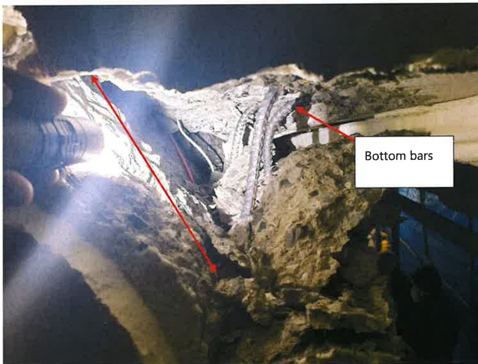
Figure 12- No Top reinforcing Steel Crossing Failure Plane. View Looking North to South at West Failure Plane. Exposed bars exposed are bottom bars.
