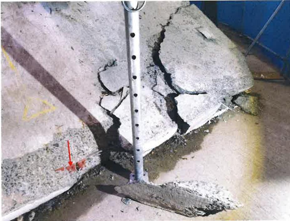
Figure 9- Live End Anchorages at East End of Lower Collapsed Slab (Red Arrow)
