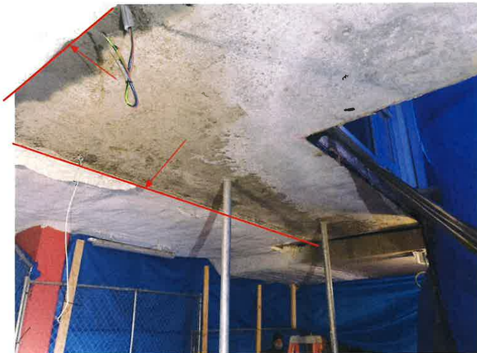
Figure 10- Formed cold joint within transition band of stepped slab, East End of Collapsed Slab
