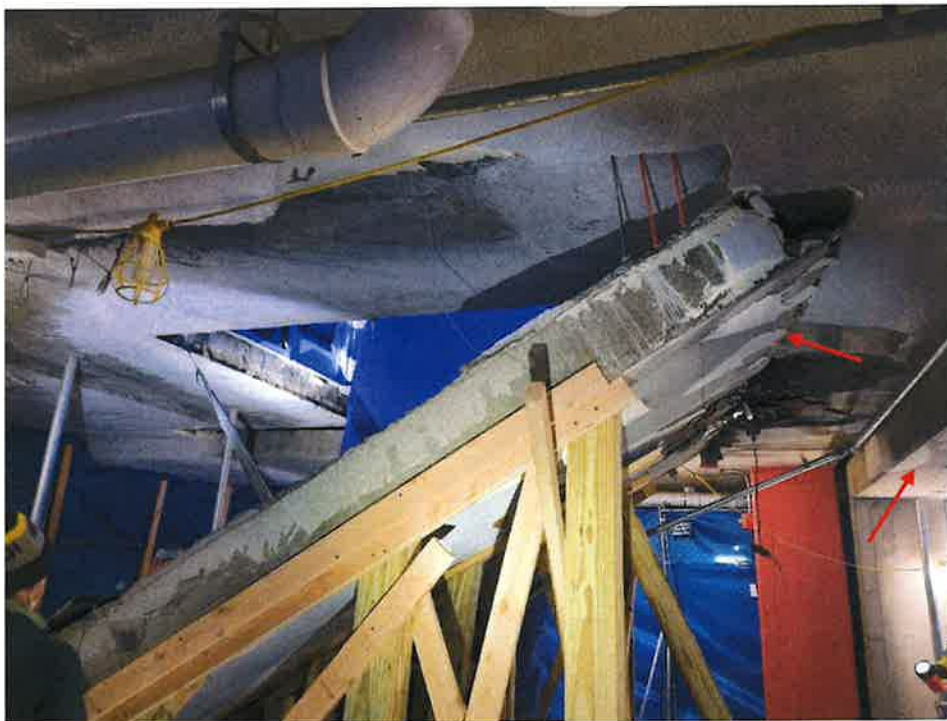
Figure 8- Shear Failure at West End of collapsed slab (left arrow). Note B21 Beam (right arrow). Collapsed Area looking South
