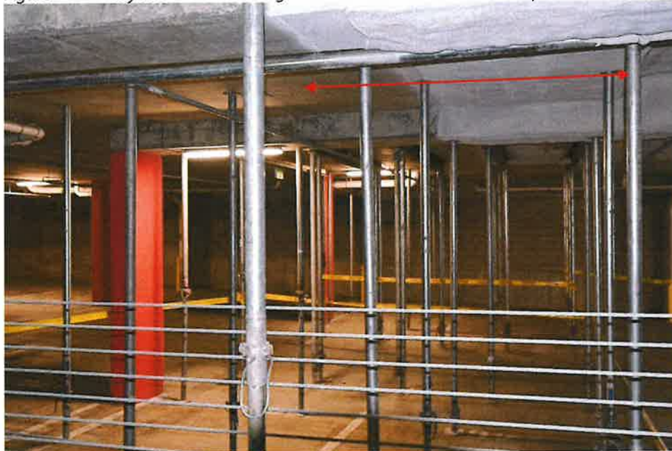
Figure 14- Underside of lower slab to west of partial collapse. Arrow indicates 83.5 in. wide region where tendons were missing in collapsed slab. WJE could not scan because of Insulation.
