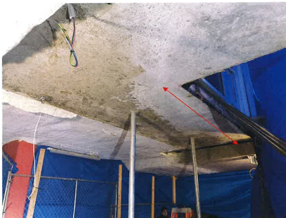
Figure 17- Upper Slab Reinforcement in the step transition Area adjacent to the Collapsed Slab is not evident (arrow band).
