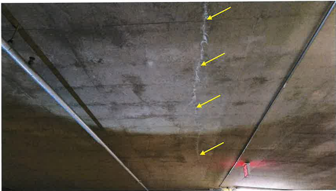
Figure 6- Typical Shrinkage Cracks at Underside of 1 st Level. Note Efflorescence Emanating from Cracks
