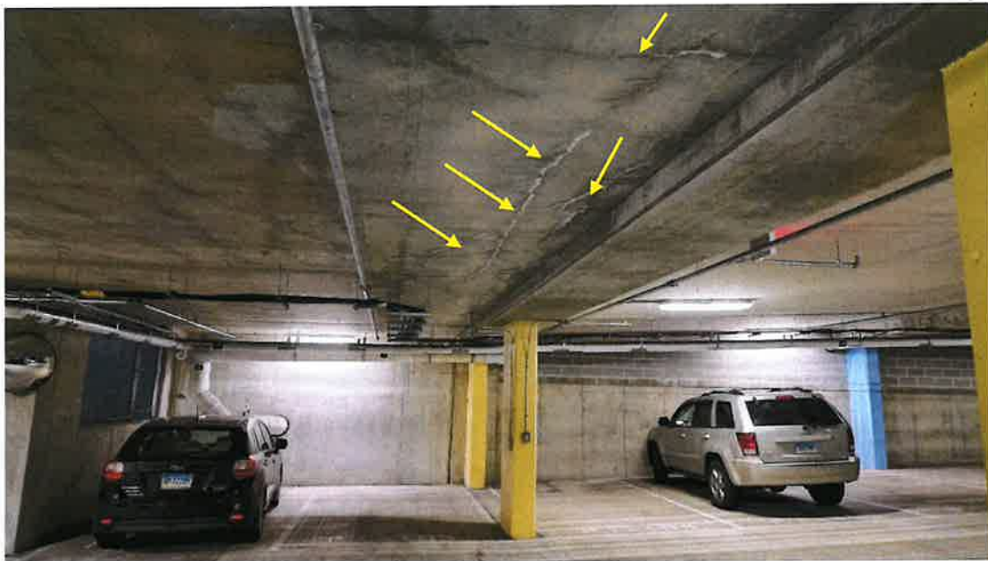
Figure 8- First Level of Garage. Note Shrinkage Cracks with Efflorescence at underside of 2 nd Floor
