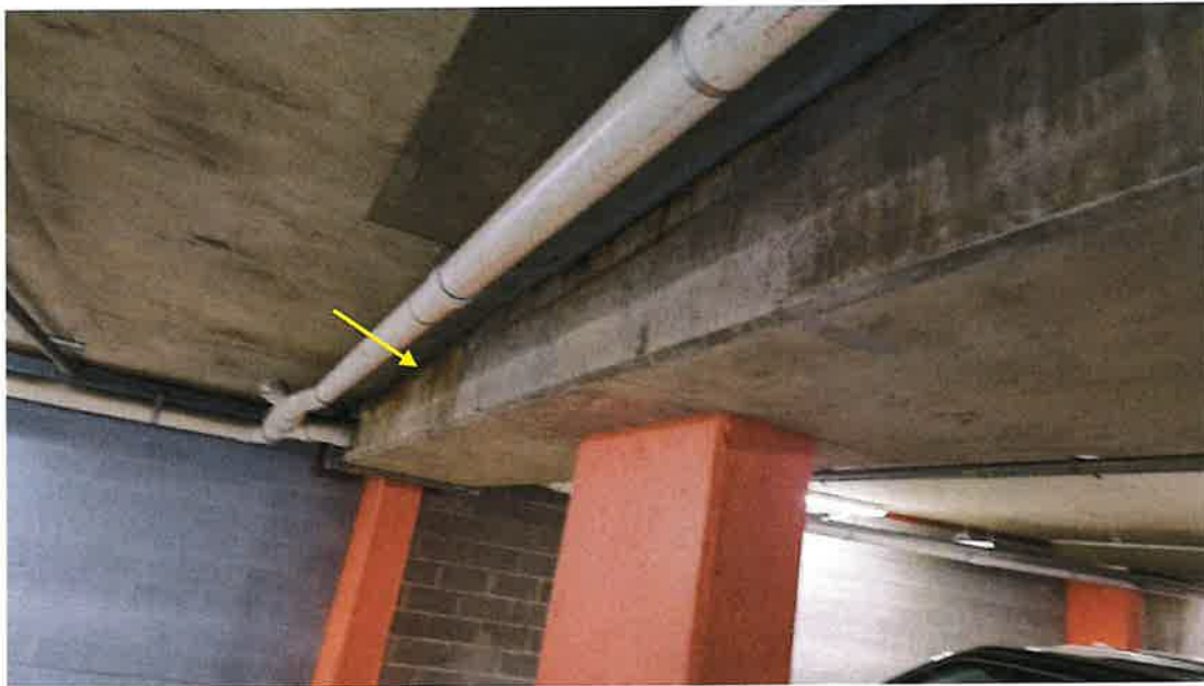
Figure 12- Corrosion at Expansion Joint
