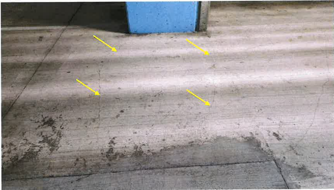
Figure 9 - Shrinkage Cracks at Floor of Second Floor Level
