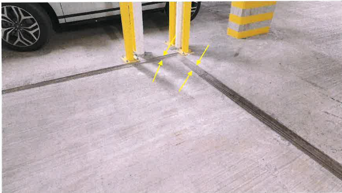
Figure 16- Deflection at Cantilevered End of Joint
