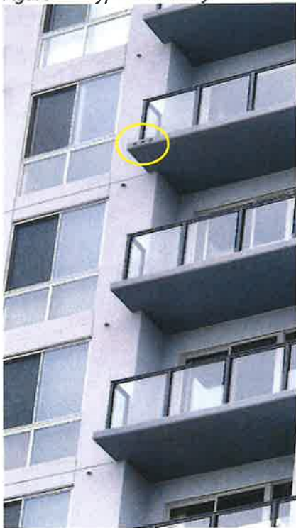
Figure 28- Missing Grout at End Anchorages
