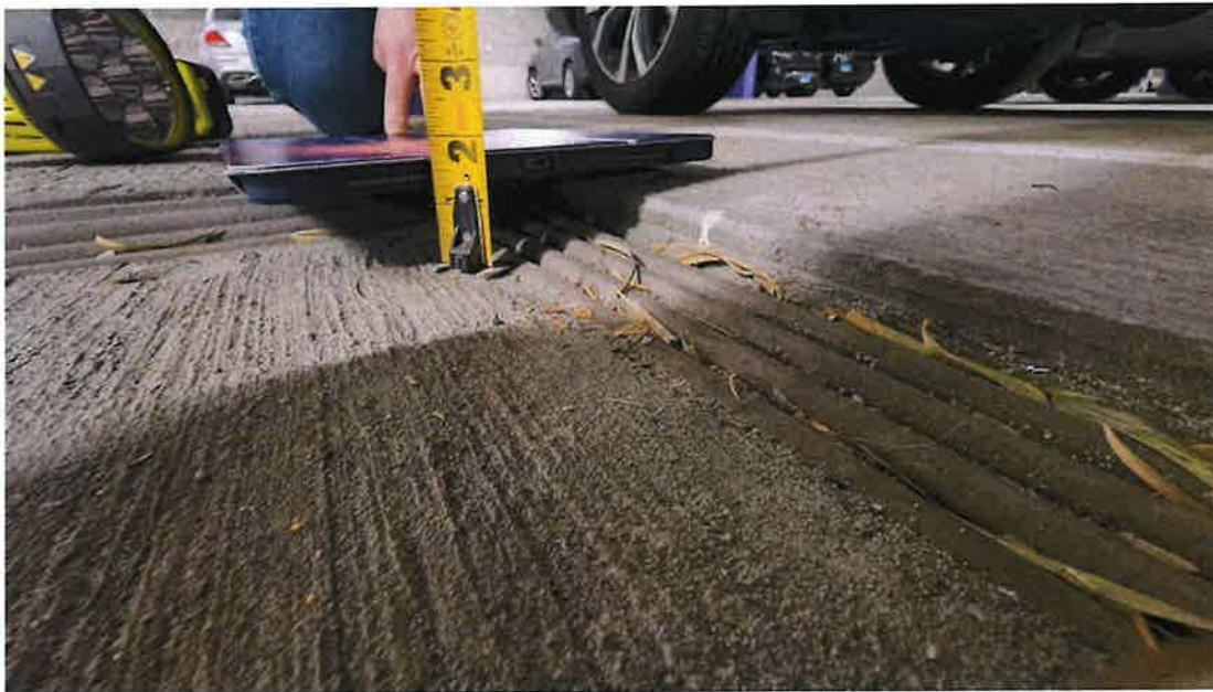
Figure 18- Deflection at Cantilevered End of Joint
