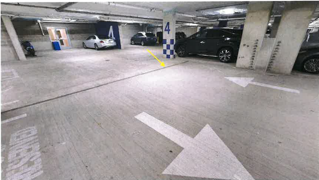
Figure 17- Deflection at Cantilevered End of Joint
