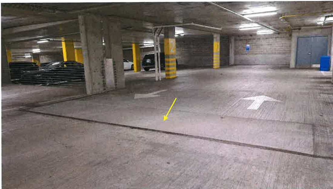
Figure 19- Repaired Expansion Joint with Plates at Underside. Note Concrete Patch.
