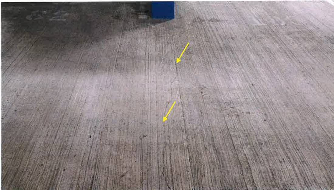
Figure 10- Shrinkage Cracks at Garage Level 1
