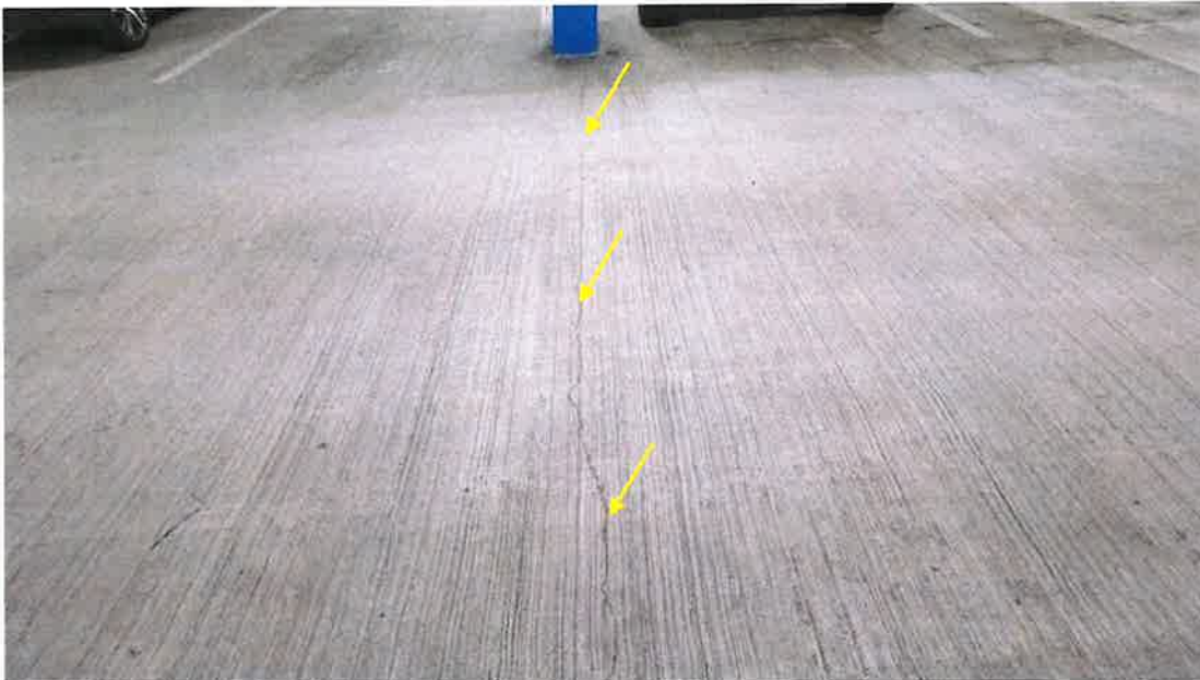
Figure 11- Shrinkage Cracks at Level 2
