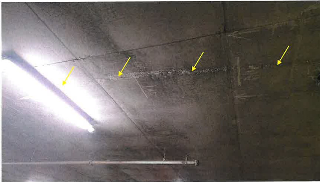
Figure 8- Shrinkage Cracks at Underside of Level 1 with Efflorescence
