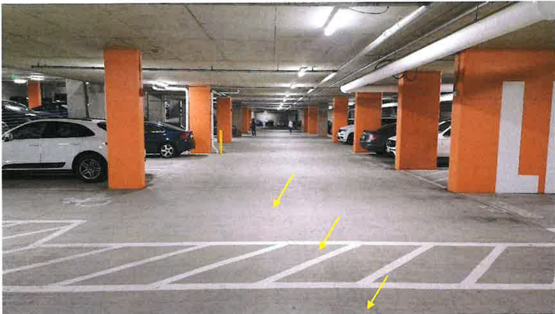
Figure 7- Lower Level of Garage, Note Shrinkage Cracks at Slab-on-Grade
