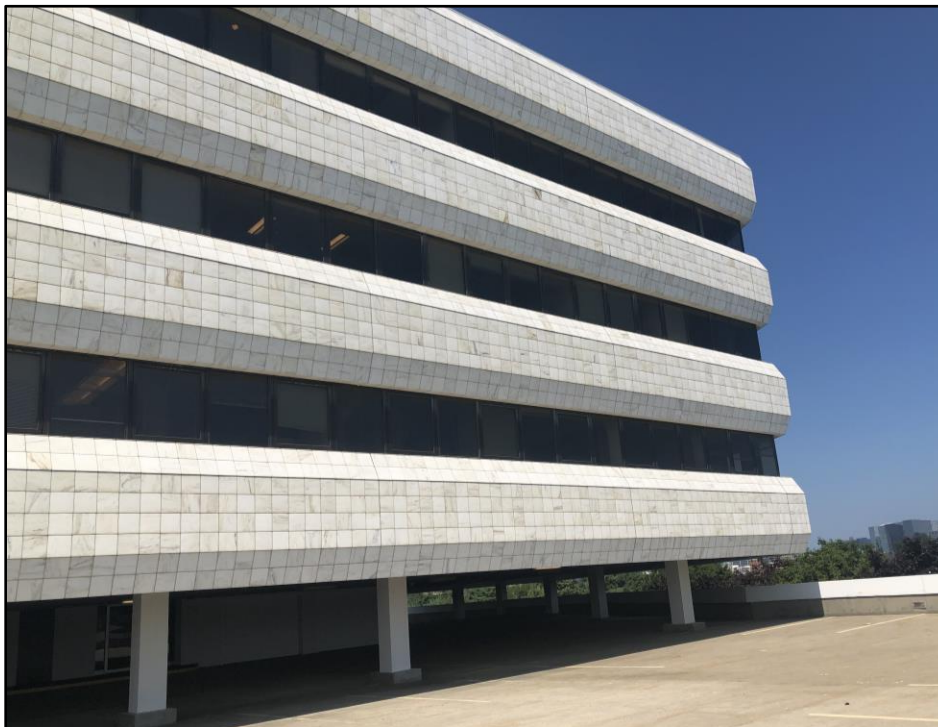
Photo 2: View of floors five through seven taken from fourth floor parking deck.
