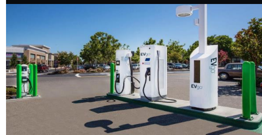
Electric Vehicle Charging Stations
