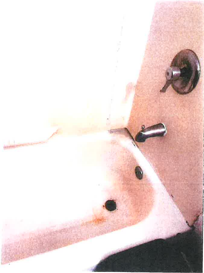
In the bathroom, the tub drain is insanitary(rusty).
