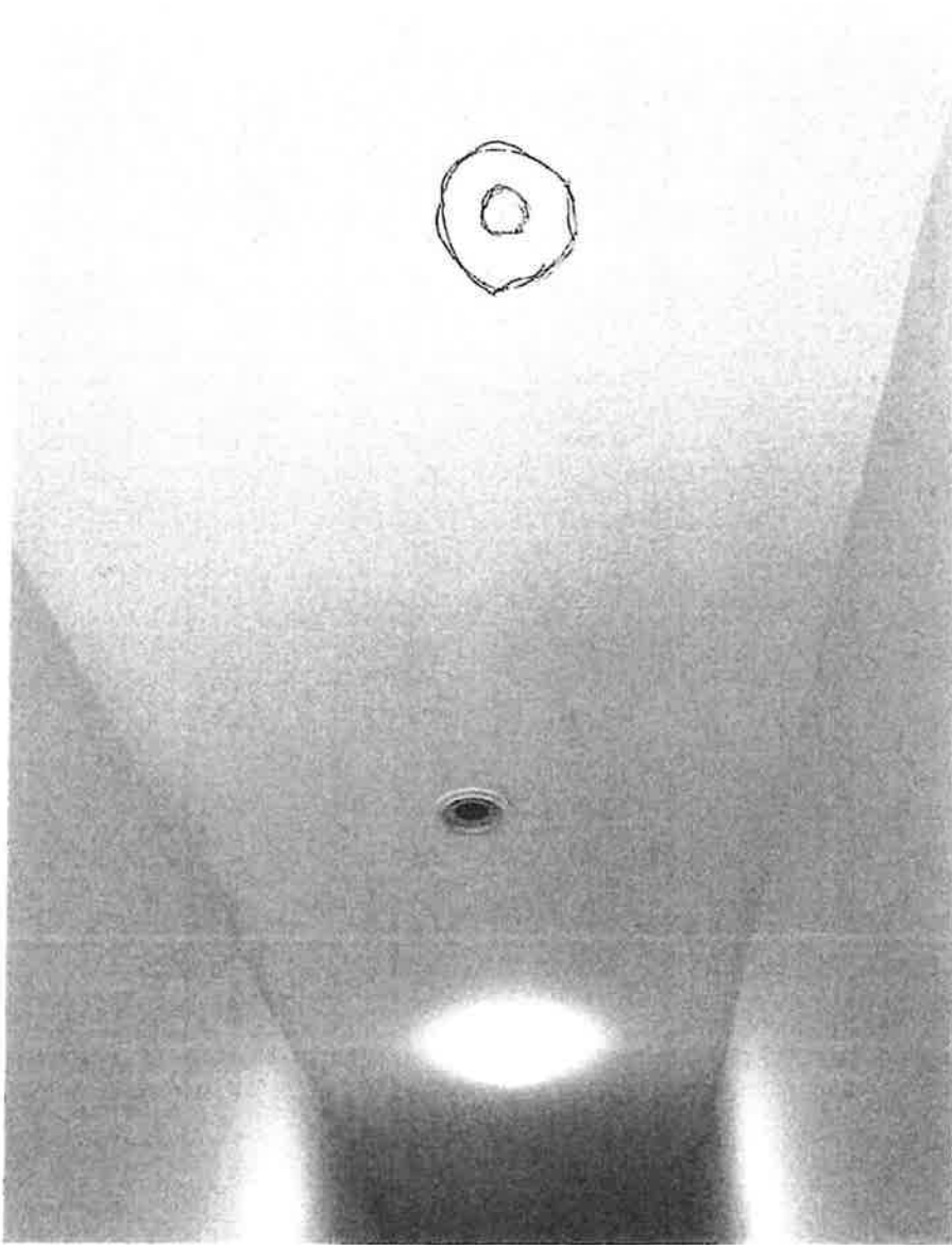
Insufficient smoke detectors
