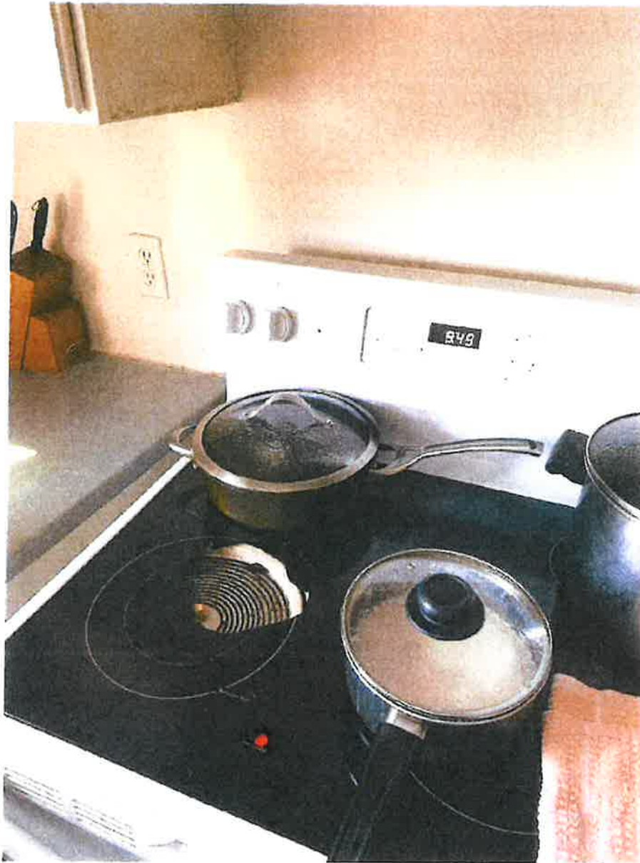
In the kitchen, the stove left front burner is in disrepair.
