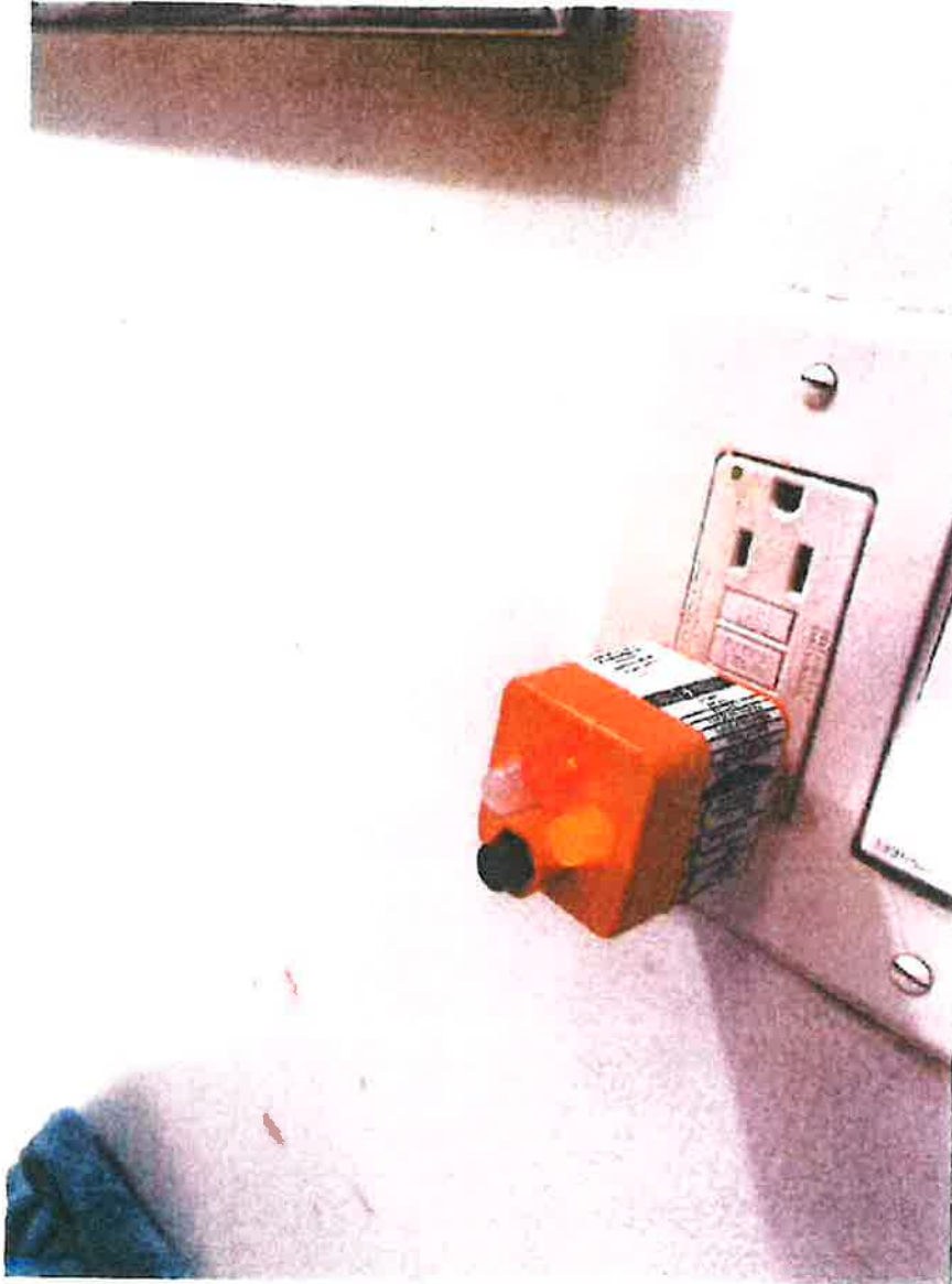
In the rear right bedroom, the electrical outlet is not working.
