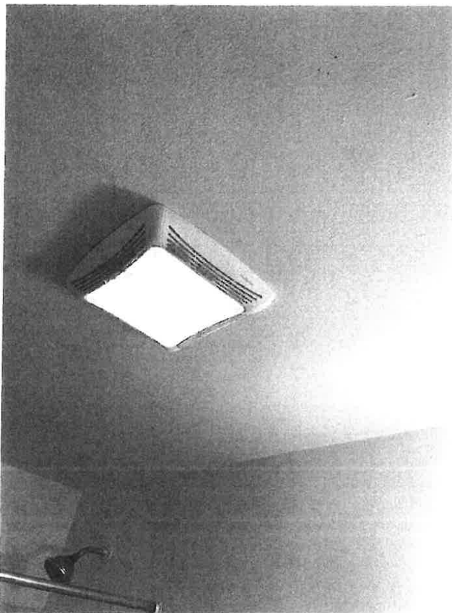
In the bathroom, the vent is insanitary.
