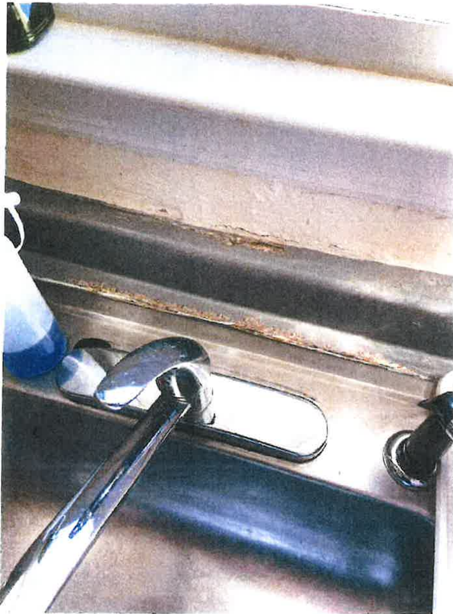
In the kitchen, the sink faucet is loose.
