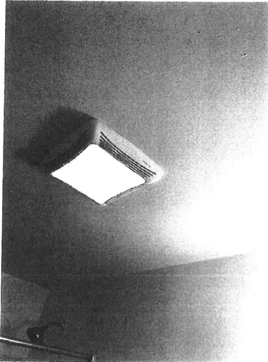
In the bathroom, the vent is insanitary.
