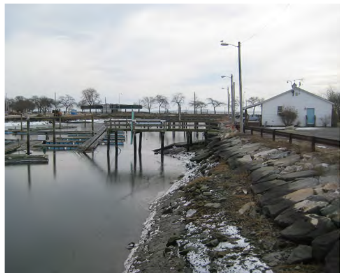
Cummings Park Marina in damaged condition following Sandy in 2012.
