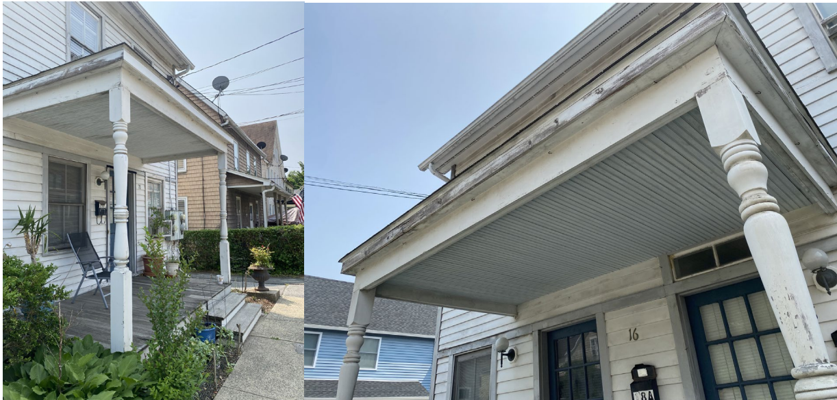
Fig. 4 (left) and Fig. 5 (right) in situ veranda posts and beadboard on the porches of 18 Taylor Street. Period-appropriate colors and finishes will be used in the restoration of the building's original porches.
