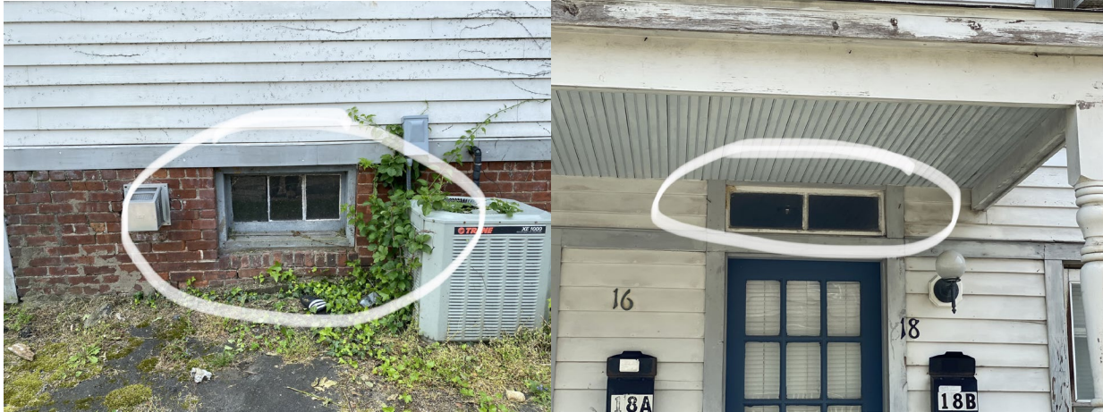
Fig. 2 (left) and Fig. 3 (right) original, in situ windows above front doors and at basement level
