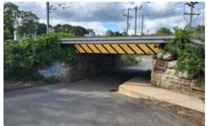
The “Cattle Crossing” (shown above) is a primary flood pathway, as the existing physical conditions are challenging.
