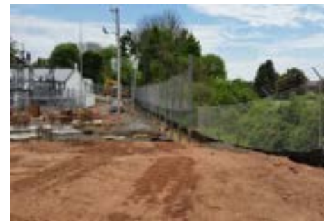
CT Statewide Stormwater Permitting Completed CTDEEP General Permit for the Discharge of Stormwater and Dewatering Wastewaters.
