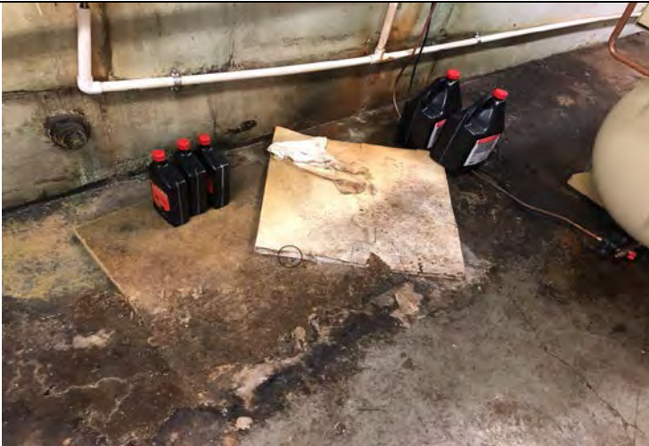
Photo 3: Staining and minor cracks in floor next to air compressor in main building boiler room. Five containers of lubricant.
