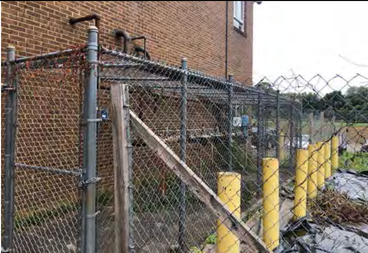
Photo 35: Main gas feed in northeastern portion of the site.
