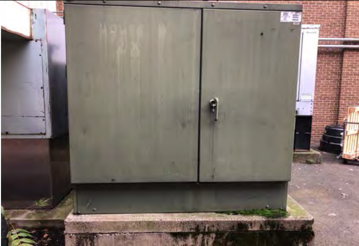
Photo 31: Transformer located in the northern portion of the site.
