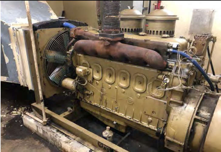
Photo 7: Diesel-fueled generator in main building.
