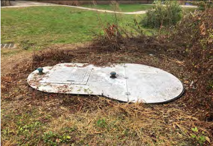
Photo 43: Sewage holding tank outside of the new vocational agricultural building.
