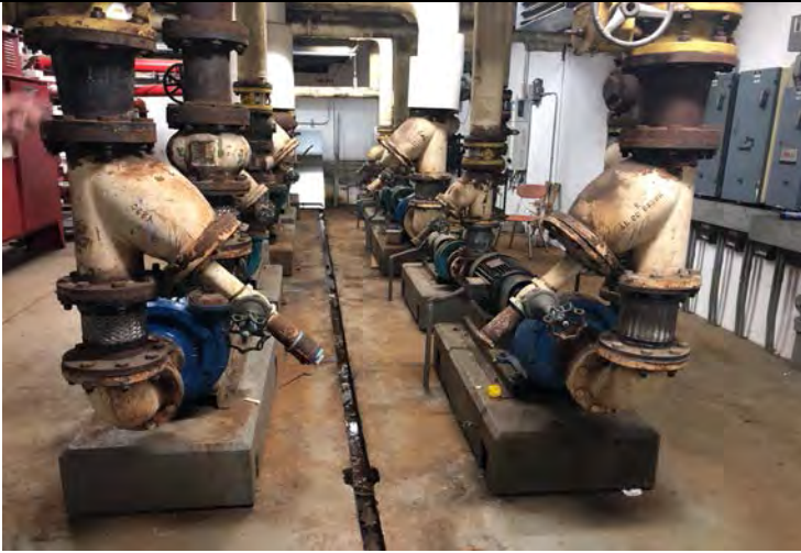
Photo 5: Main building boiler room pumps.
