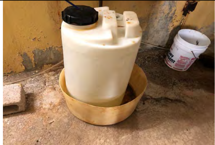
Photo 24: Muriatic acid tank in pool mechanical room. Tank in secondary containment.
