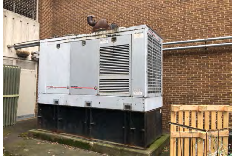
Photo 30: 500-gallon diesel-fueled generator located in the northern portion of the site. Used to power the fire pump system.
