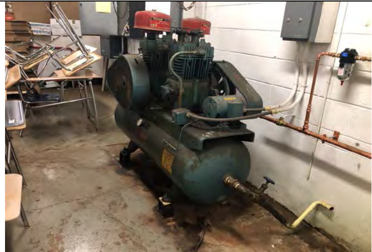
Photo 4: Air compressor in main building boiler room.
