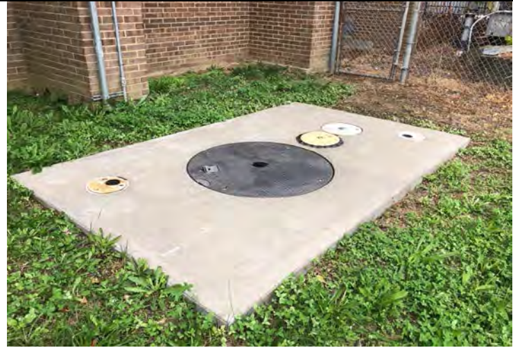
Photo 6: 500-gallon diesel fuel UST.
