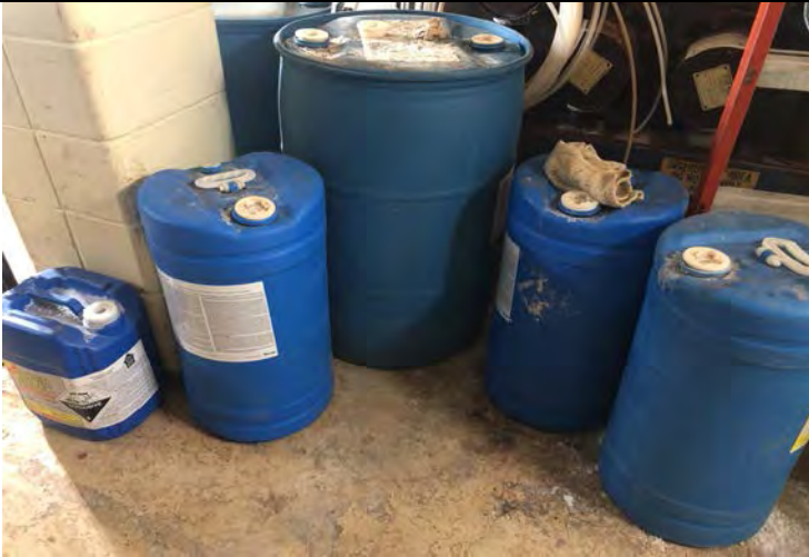
Photo 23: Containers of chlorine in pool mechanical room.
