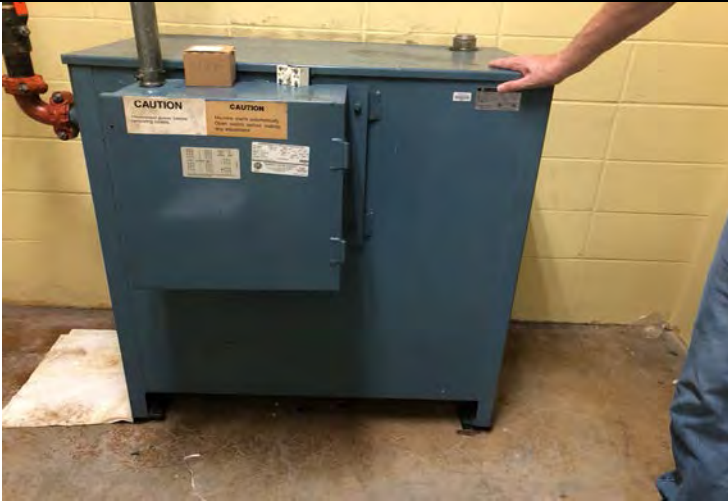
Photo 39: Hydraulic tank in one of the elevator machine rooms in the main building.
