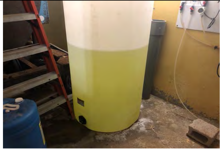
Photo 22: Leaking chlorine tank in pool mechanical room.
