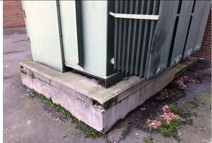
Photo 32: Transformer located in the northern portion of the site.
