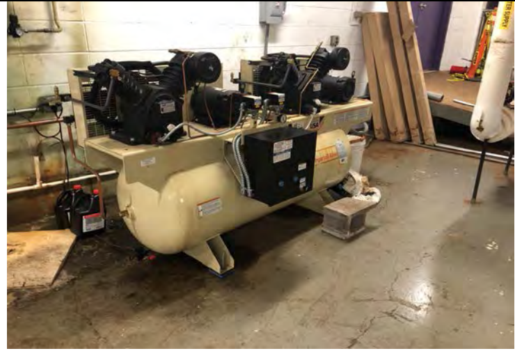
Photo 2: Air compressor in the main building boiler room.
