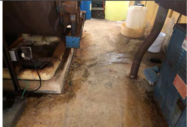
Photo 20: Water leaking from pipes in pool mechanical room. Water flowing into a floor drain.
