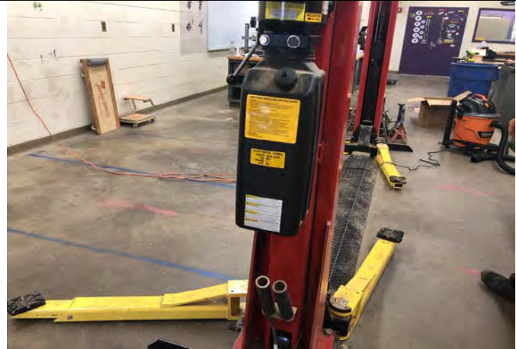
Photo 12: Above-ground lift in automotive shop.
