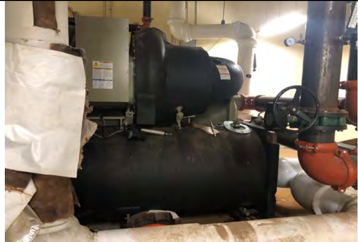
Photo 8: Old chiller no longer in use in main building.
