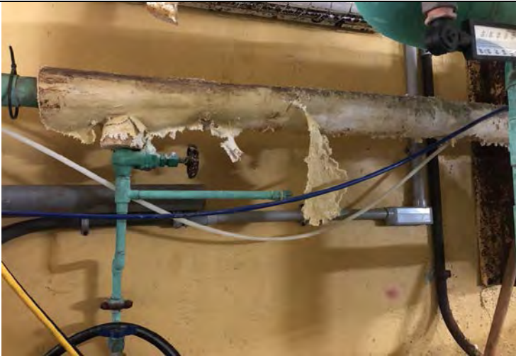
Photo 19: Pipe wrap in pool mechanical room
