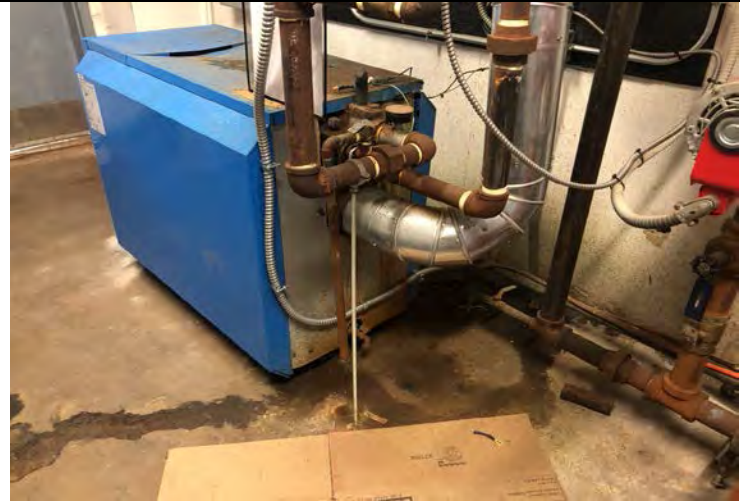
Photo 48: Boiler in the old vocational agricultural building. Visible staining on the ground.
