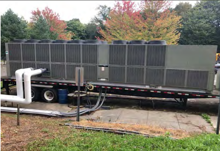
Photo 11: Current cooling system located on the western portion of the property.
