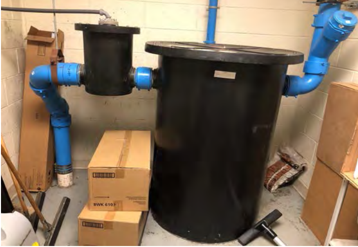
Photo 29: Waste acid tank for used classroom chemicals. Located on the first floor near classrooms numbered in the 500s.
