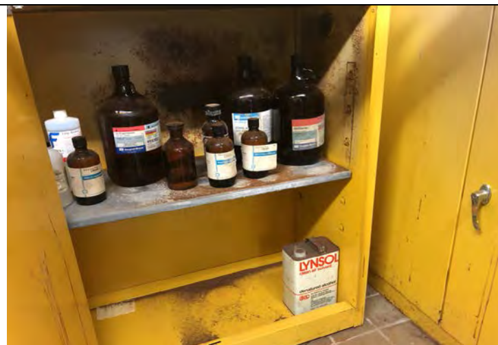
Photo 28: Chemical storage and prep room flammables cabinet.
