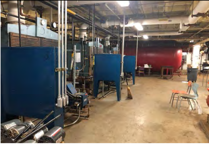
Photo 1: Main building boilers and fire pump system.
