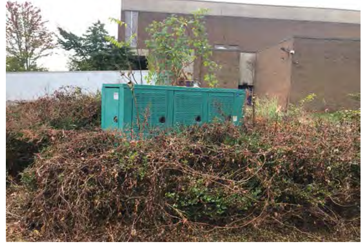
Photo 42: 170-gallon generator outside of the new vocational agricultural building.
