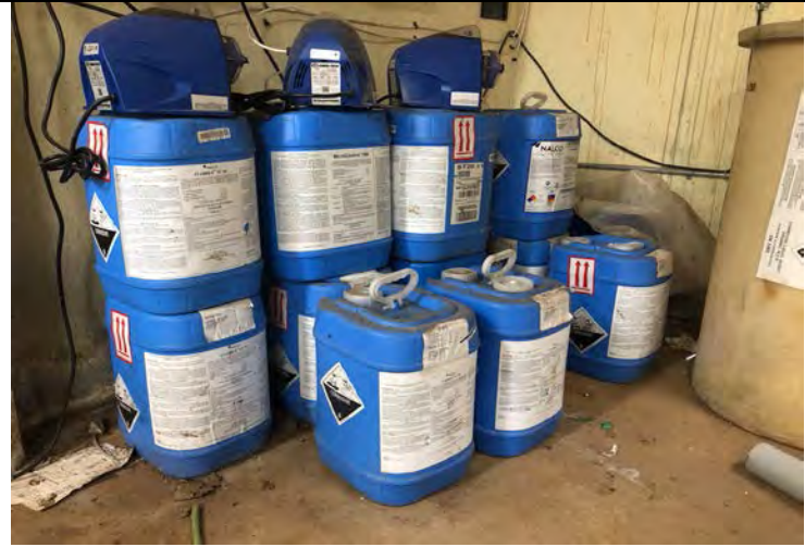
Photo 10: Eleven containers of Stabrex ST20 anti-bacterial chemical for old chiller in main building.
