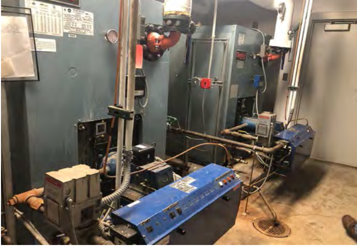
Photo 41: Boilers in one of the two boiler rooms in the new vocational agricultural building.
