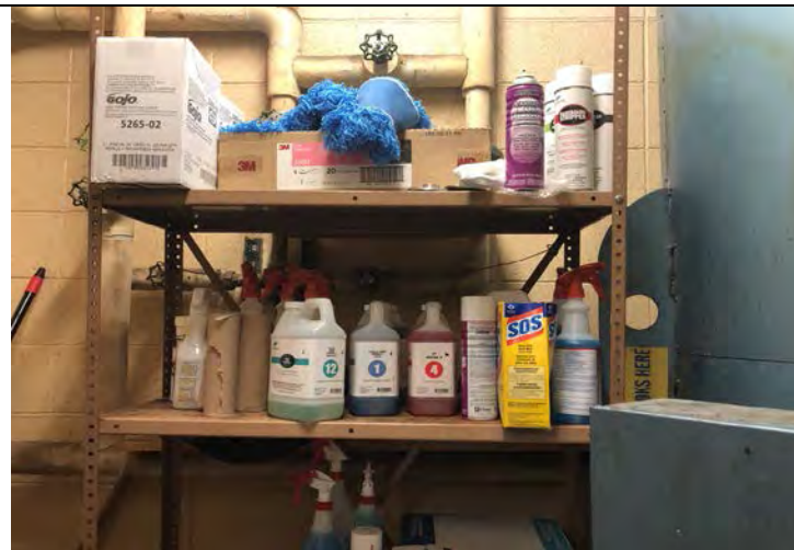
Photo 26: Janitor's closet cleaning supplies and electric water heater.
