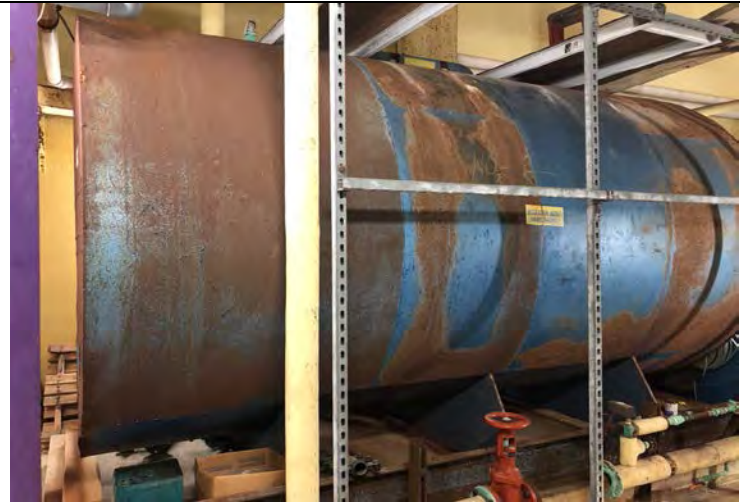
Photo 18: Old pool water heater (no longer in use) in pool mechanical room.
