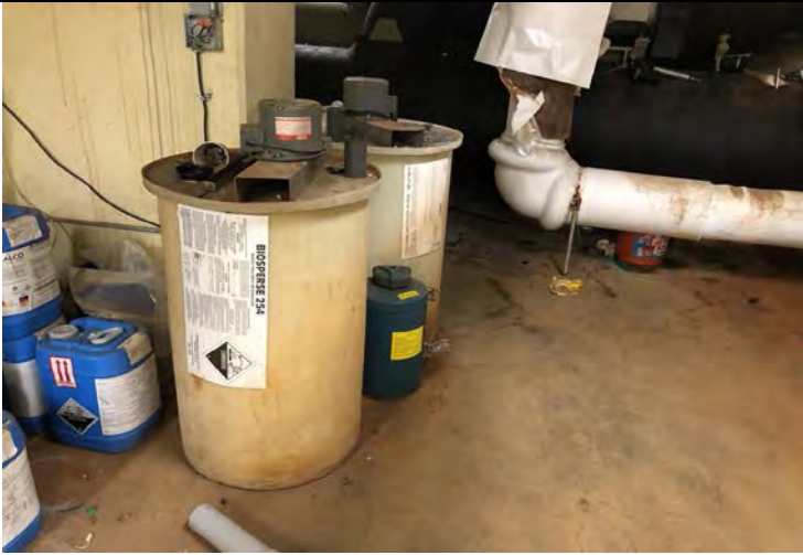
Photo 9: Two containers of Biosperse 254 microbiocide next to old chiller in main building.
