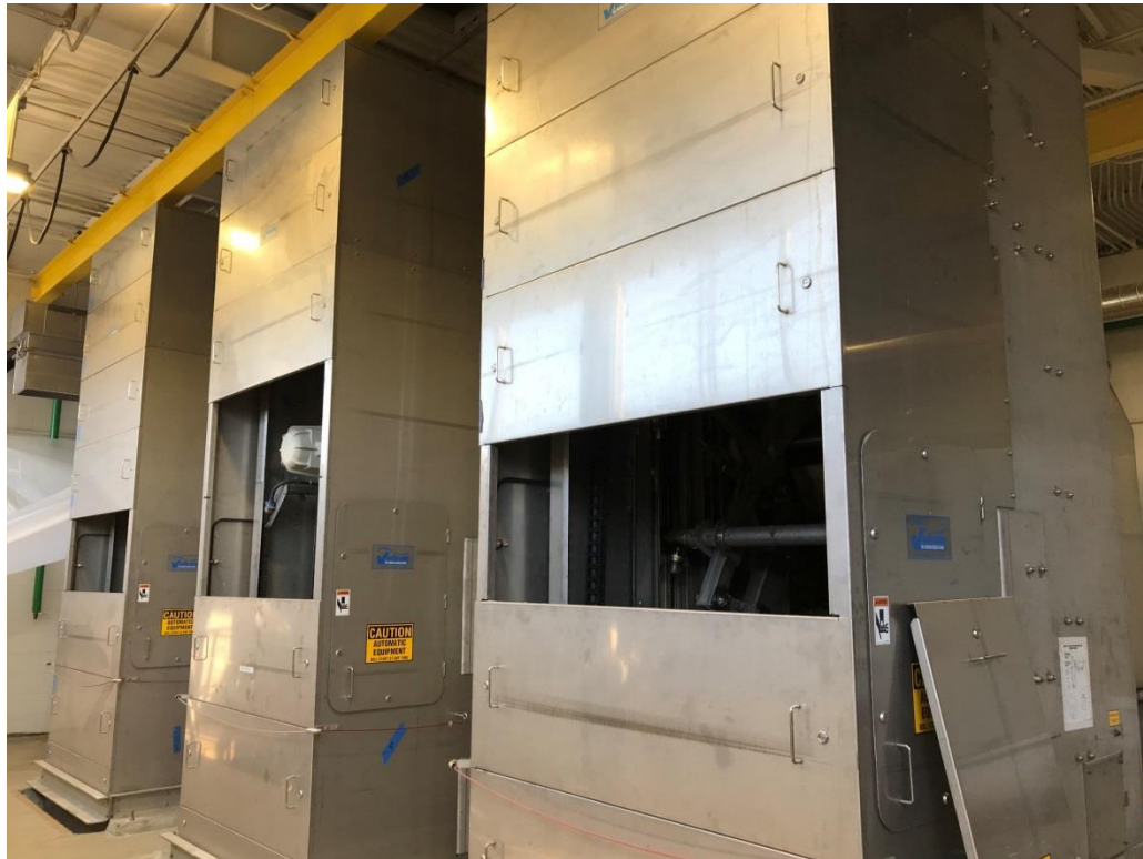
New Mechanical Screens
