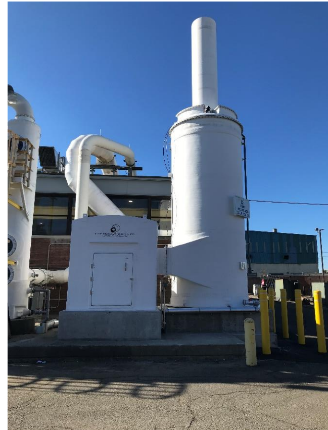
New Odor Control
